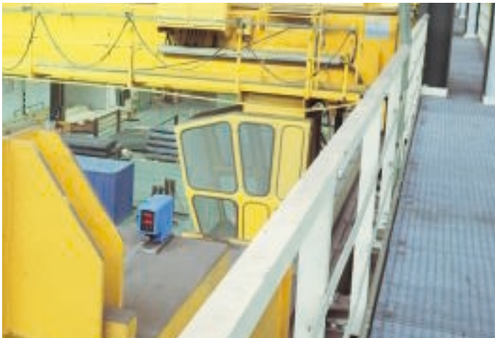
▲ Crane monitoring with DME: The distance measuring device triggers the emergency stop when a minimum distance is undershot.
